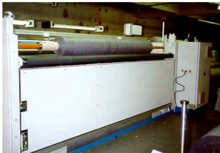
Fig. 3: View with partial capsuling in the rear operating passage with web lap
